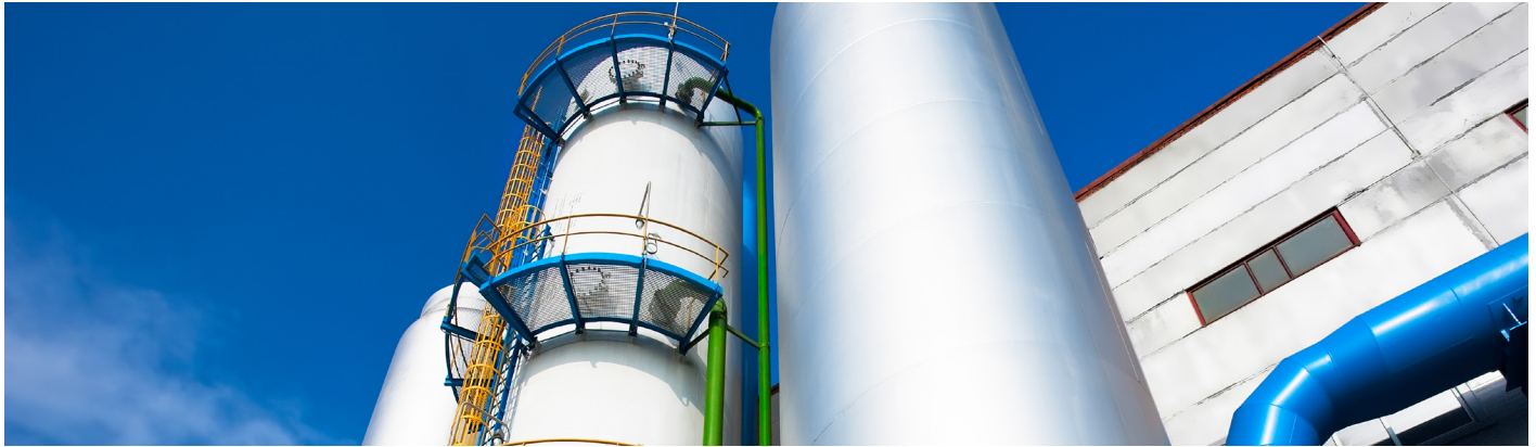
Air Separation Plant
